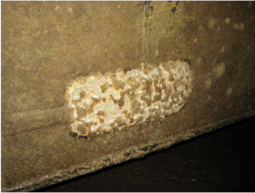
Spent anodes that require replacement.
