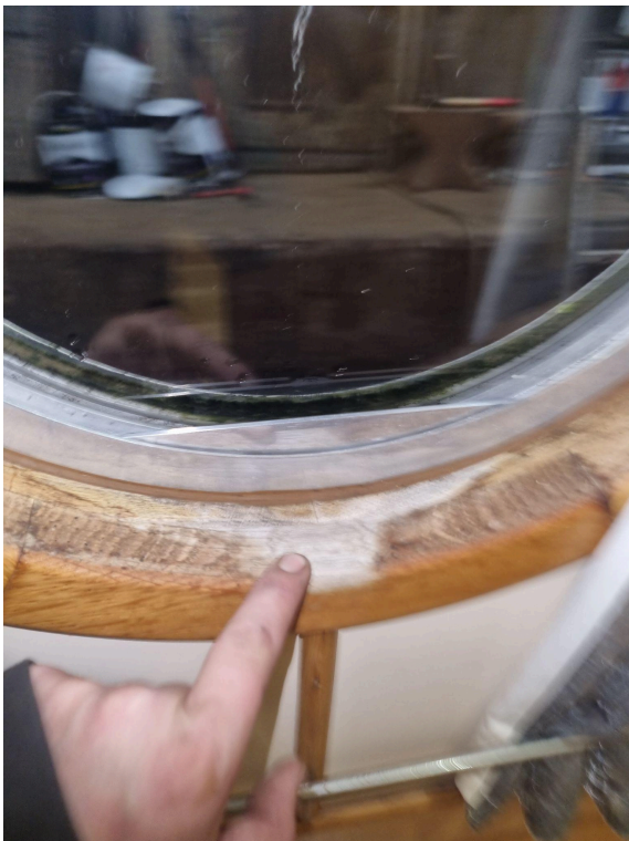
Watermarks beneath windows
