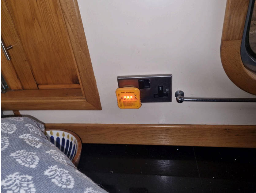
Socket outlet test
