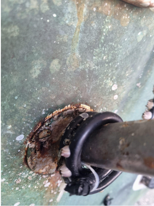
Bathing platform strut fixings with pitting and a cable wrapped around it.
